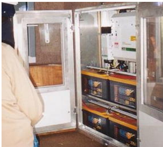
4 leisure batteries and an inverter in a vehicle with pv panels and a wind turbine
