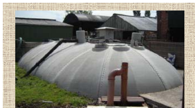
larger-scale digester on a dairy farm in Shropshire; built by Farmgas (who have built many agricultural digesters). It is about 15 years old and still operational.
