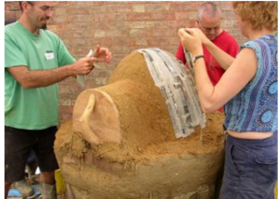
covering a dome of damp sand (with wooden door attached) with wet newspaper; the oven will be built around this, and then the sand scraped out to form the chamber
