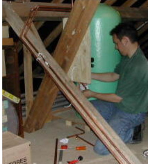
installing a twin-coil cylinder with pump & control set (for solar hot water) in a loft, with copper pipework and 45° elbows
