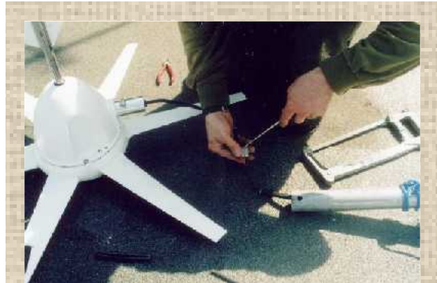
installation: the installer is here connecting the wires that run down the mast to the batteries and inverter. The wind gen will then be fixed to the mast, and the mast raised and fixed in place with guy wires.
