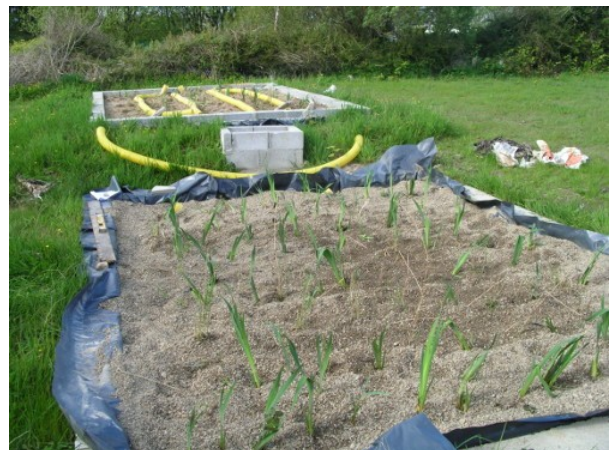
Reed bed mid-construction: upper vertical flow bed followed by lower horizontal flow reed bed, then planted with Phragmites and Iris.
