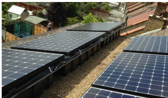
2kW installation on a flat roof in London.
