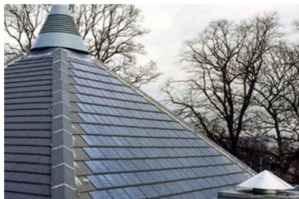
Solar roof tiles on a roof in Nottingham.
