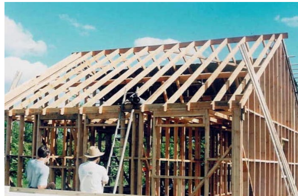
Finishing off the stud frame, onto which will be fixed insulation, exterior cladding, interior walls and roofing material.
